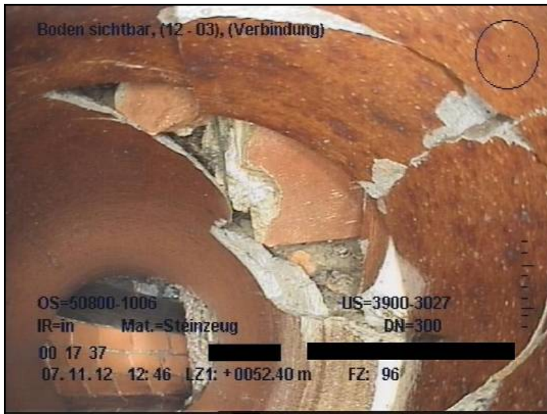
Baulicher Mangel [Rendsburg, 2014]
